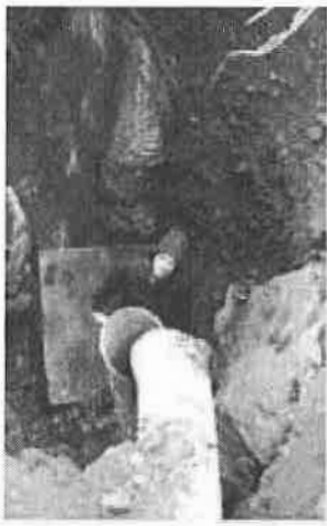
Fig. 37. (Above) A large sinkhole collapse around a poorly installed drainage well.
