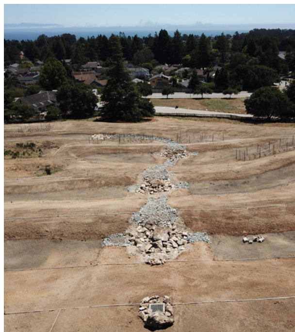
▲ Stormwater management at Emergency Response Center
