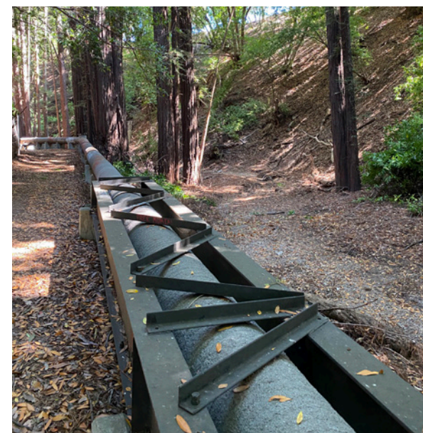
▲ Jordan Gulch above grade sewer
