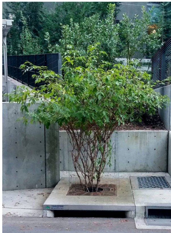
▲ Biomed Stormwater Treatment
