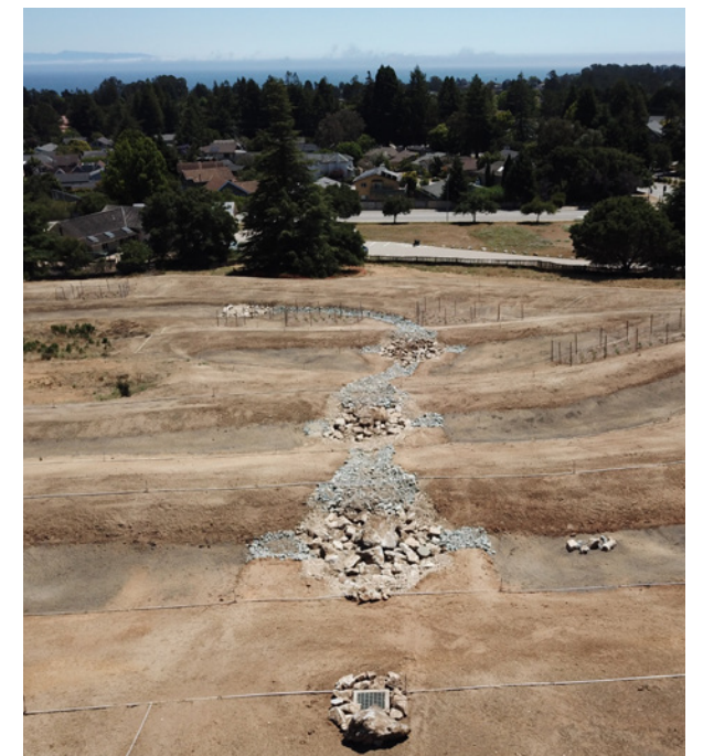
▲ Stormwater management at Emergency Response Center
